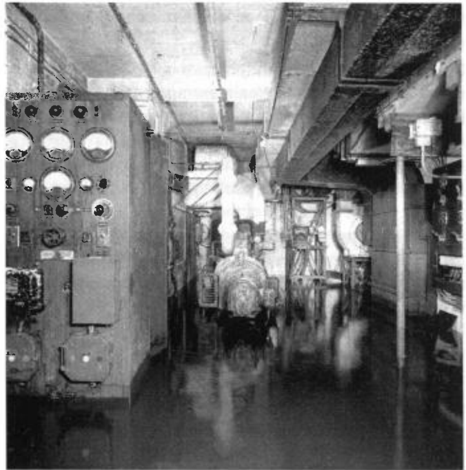
The standby generator
